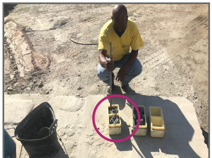
● In the above photograph plastic moulds are in use and to avoid damaging the cube a steel rod is being used for compaction. The effective compaction (and strength) of cubes under such circumstances is suspect.
